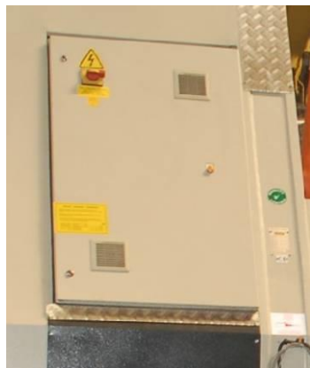
MAIN SWITCH WITH DOOR INTERLOCK
